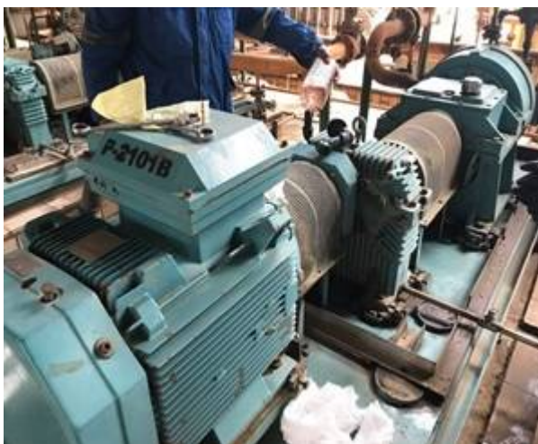
Fig. 6 Oil injection in pump gearbox P-2101 Fanavaran petrochemical company
