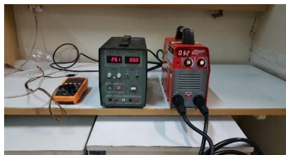
Fig. 9 Electric current supply equipment to generate magnetic field and current applied to the fluid
