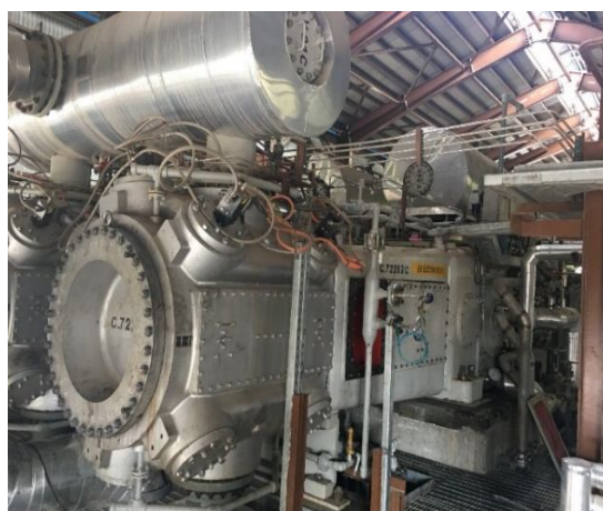
Fig. 1 Neuman Esser horizontal reciprocating compressor
